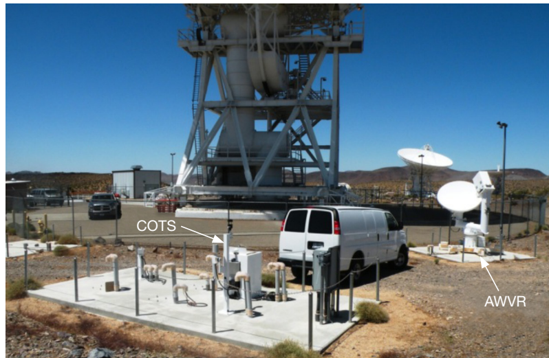
Figure 6. COTS and AWVR instruments installed at DSS-25.
