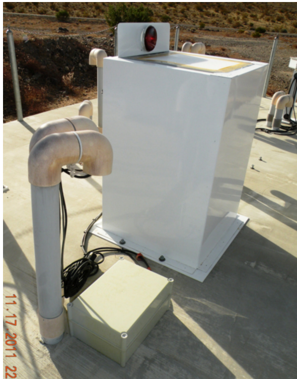
Figure 4. Radiometer in enclosure installed at DSS-25.
