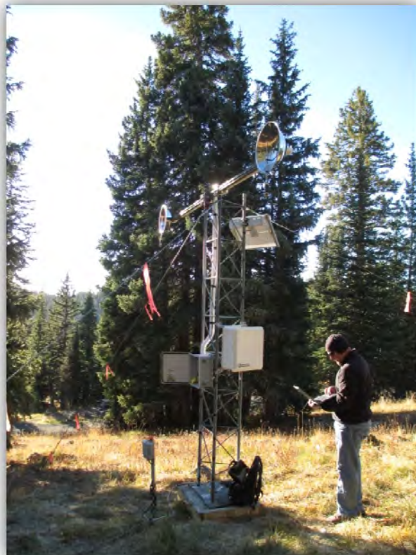
Figure 9. DRI Weather Station (Courtesy DRI)
